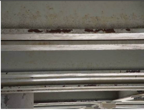
Figure 15. Duplex TSZ failure on catch frame
