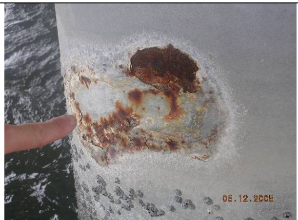
Figure 14. Failure of TSA repair
