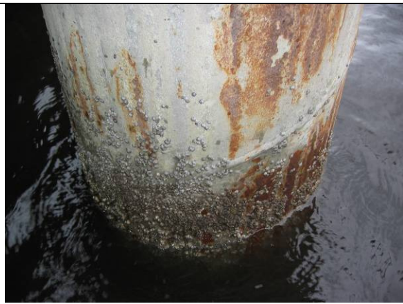
Figure 12. TSA “failure” on pile
