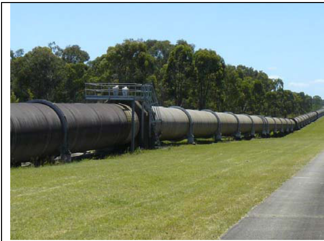
Figure 7. Warragamba Pipeline (P2)
