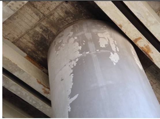
Figure 16. Seal coat delaminating on TSZ
